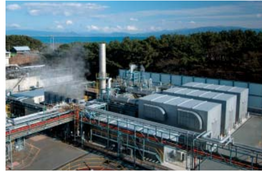
Natural gas engine cogeneration facility at Polyplastics Co., Ltd.'s Fuji Plant
